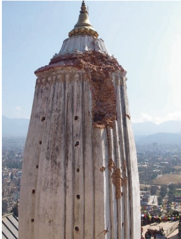
Fig. 5.3 Lightning damage to a historic temple in Nepal. (Courtesy Shri Ram Sharma)
