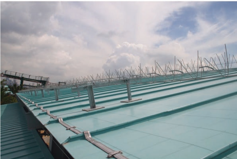
Fig. 17.6 “Lightning eliminators” – not accepted by any lightning standard. (Courtesy of HCFP Pte. Ltd.)
